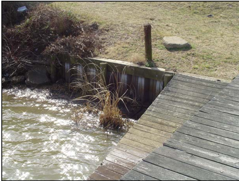
Retaining walls and rip rap to control erosion at Port Royal Boat Landing
